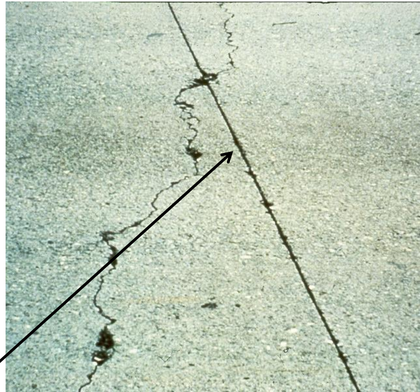
This one was sawed too late
