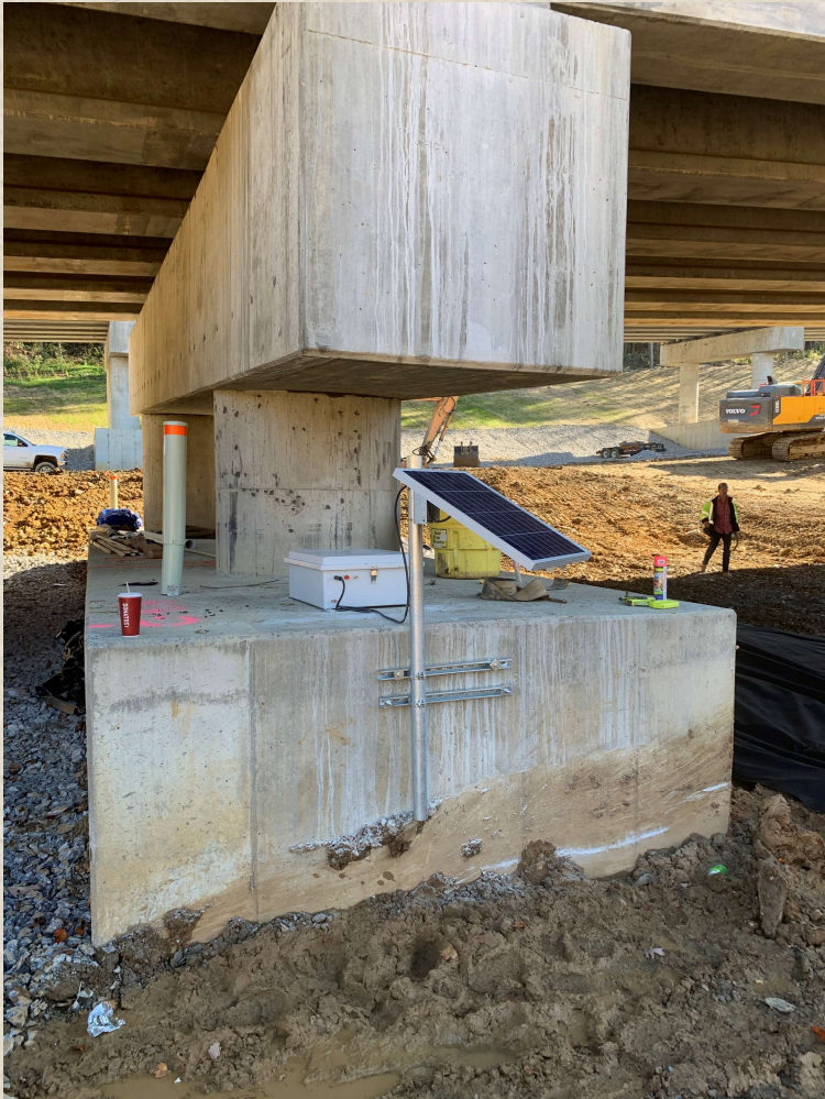
Star Hub and Solar Panel
