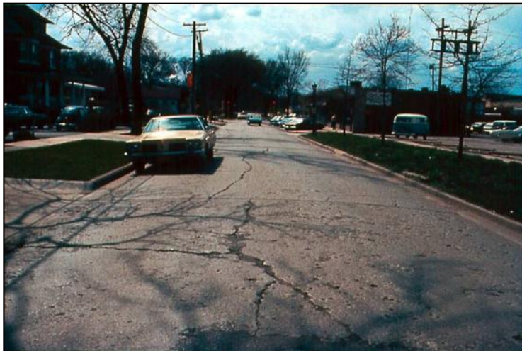
Erratic crack patterns due to no joints
