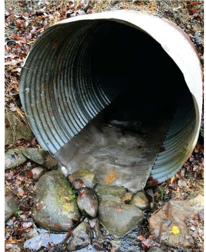
Concrete Cloth lining of a corroded culvert in Seymour, TN with an active stream
